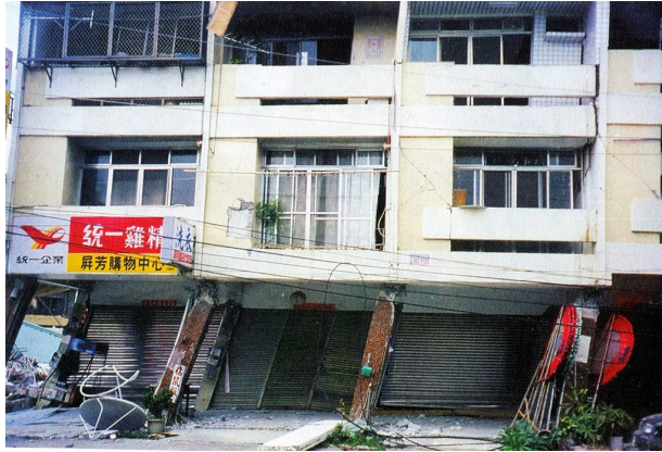
Fig. 2. Failure of the first story of row houses along the street direction during the 1999 Chi-Chi earthquake
